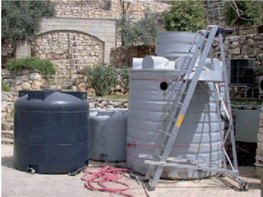
Figure 16.4 Aerobic OMW pilot (5,000L) treatment plant (LAU, Byblos Campus, Lebanon)
