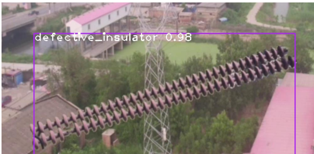
Figure 37: Defective Insulator Test
