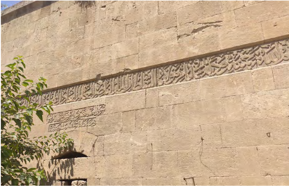
Figure 18. A section of the external inscription band on the eastern façade of madrasat al Firdaws. Picture taken by the author
