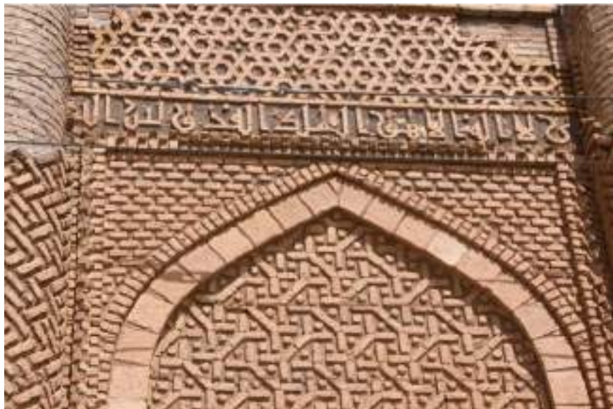
Figure 70. Detail of Kharraqān towers A.D.1067 and A.D.1093 Kharraqan region of northern Iran, near Qazvin
